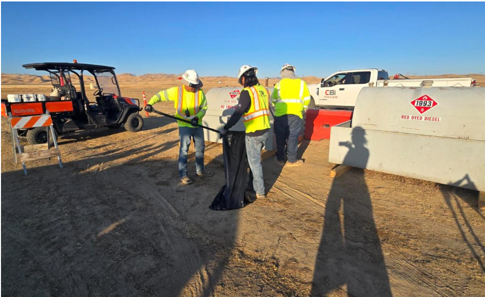
Photograph 8: CBI crew collecting contaminated soil from diesel fuel spill on 5/22/2026.
